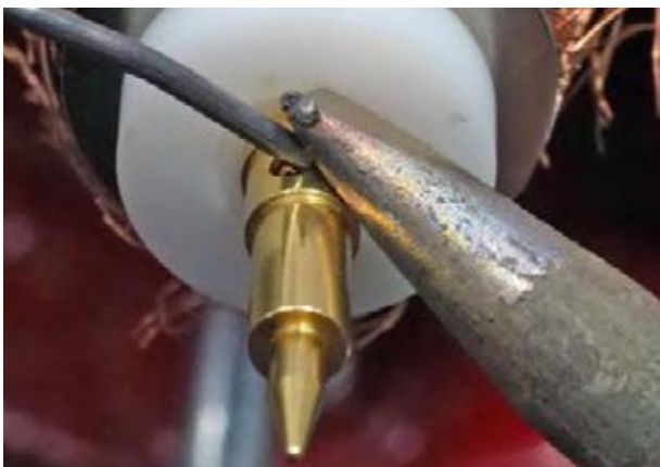
The welding must be as quick as possible: 2-3 seconds for "N" connectors.
